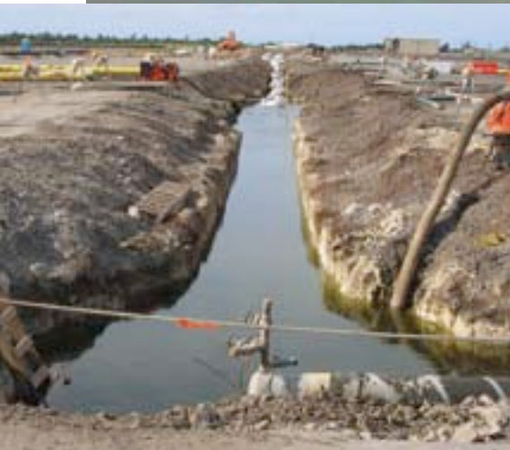
Nova Group dewatered trenches and retention ponds to build a hydrant fueling system at Hickam Air Force Base, Hawaii.
